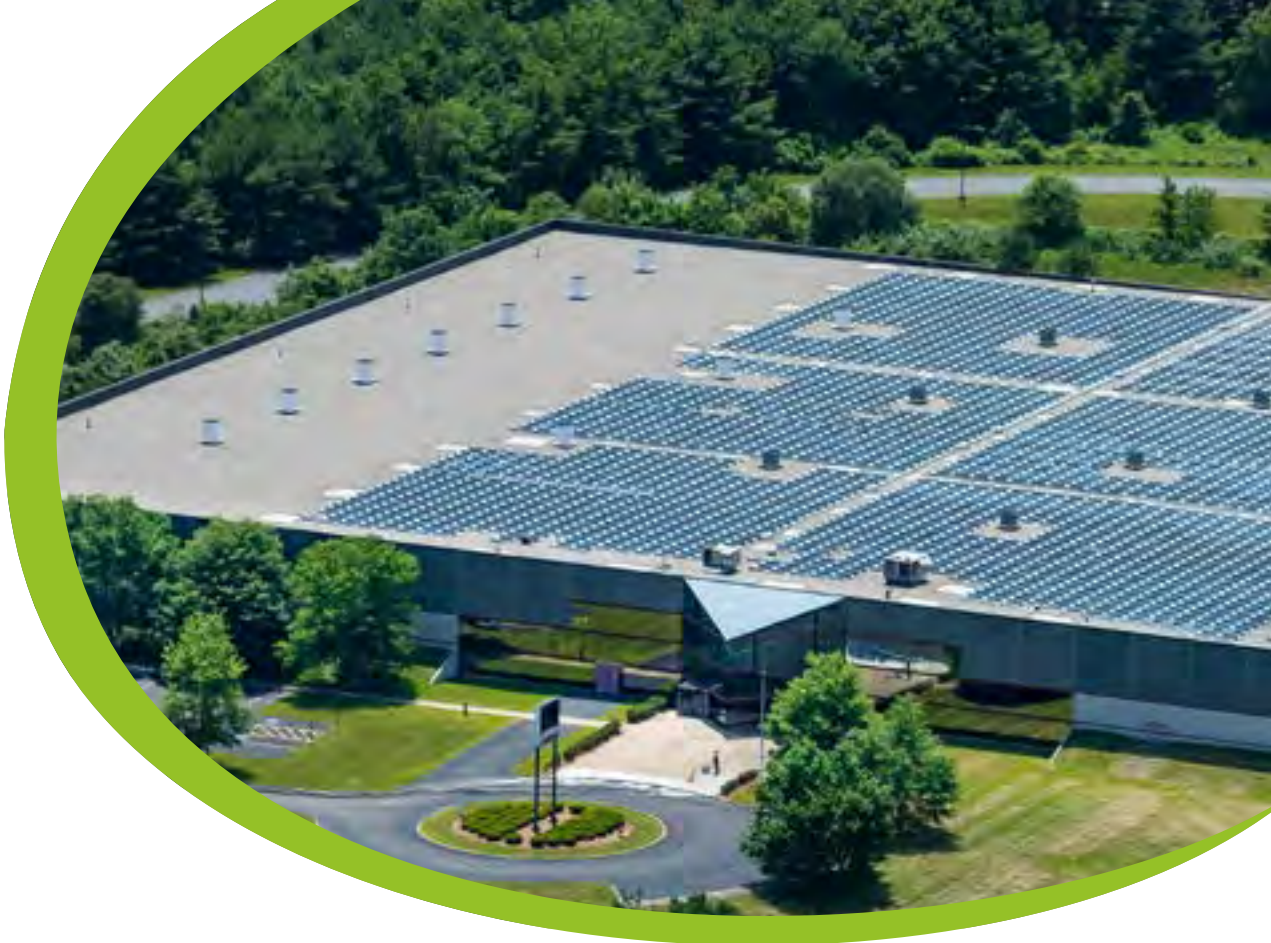
SED Solar Portfolio - rooftop solar system installed at an industrial facility in Massachusetts
