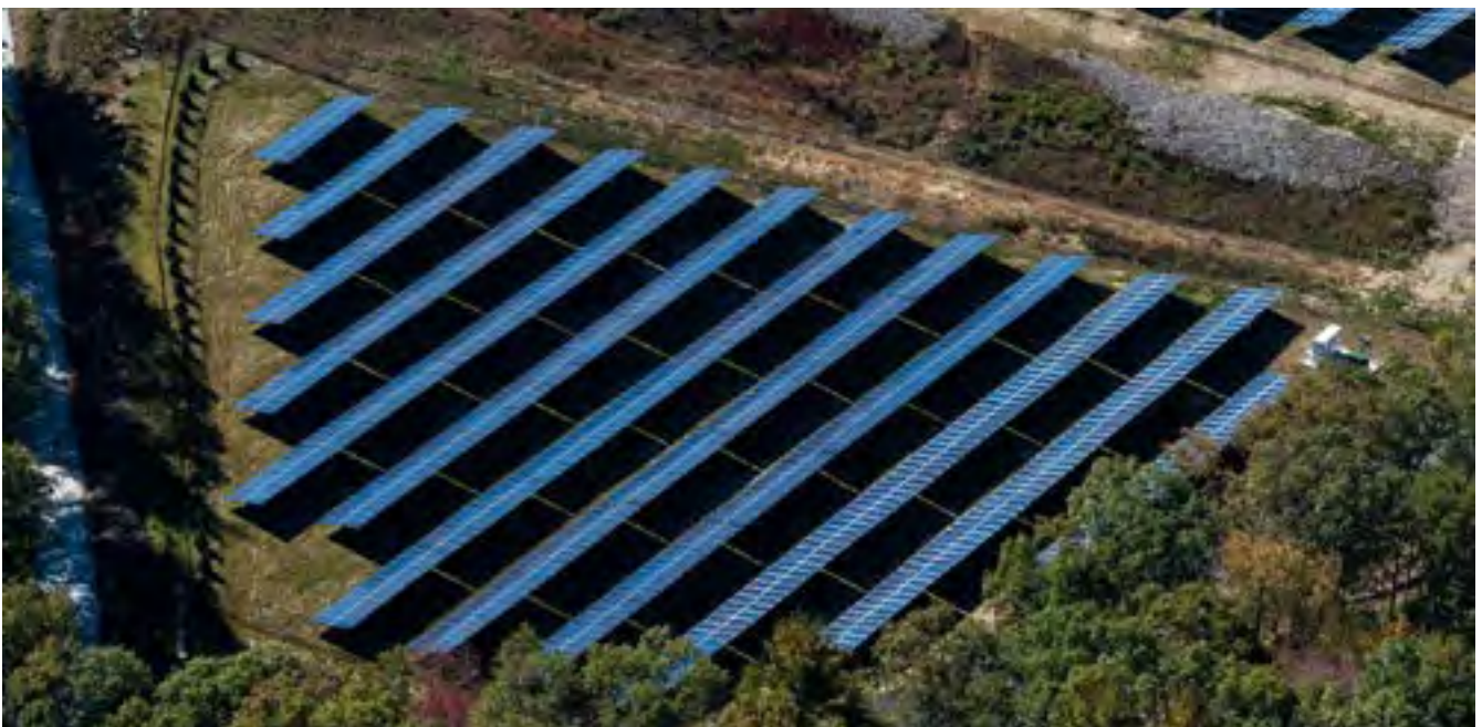
Ground mounted solar project in Massachusetts, part of the SED Solar Portfolio
